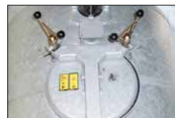
Ø 600 mm upper manhole on hinge
