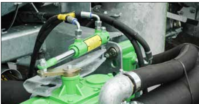
Hydraulic pump change-over
